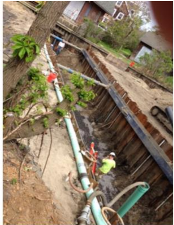
Figure 1 – Image 1: Scow Ditch dammed and drained. Photo taken standing adjacent to the south end of Fire Company parking lot looking NNE.
